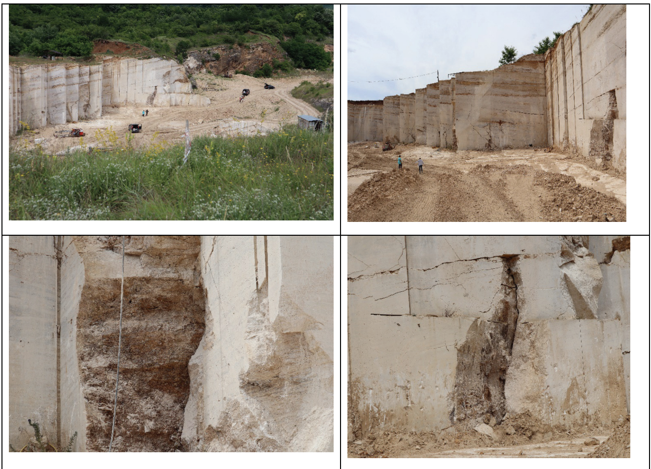
Figure 4. Cărpiniș Quarry and images of cracks. (“original”).
